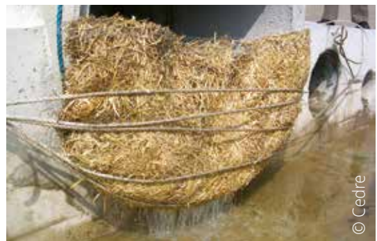
A filter cartridge installed at an outfall
