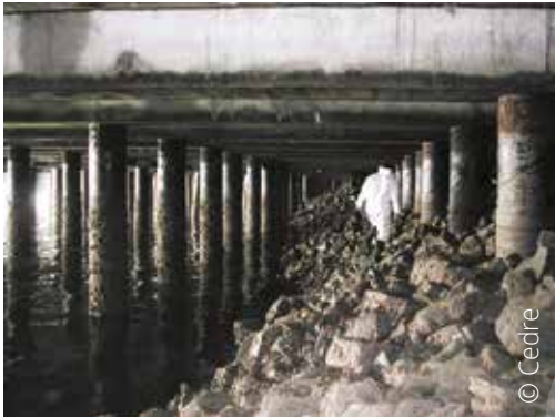
Oiled riprap and wharf pilings
