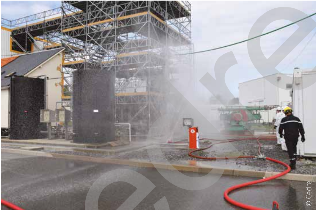
Protecting a building with a water curtain sprayed by a water shield
